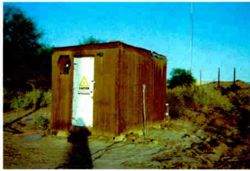
Fig. 1: The transmitter shack — complete with live AC wiring running along the ground.
