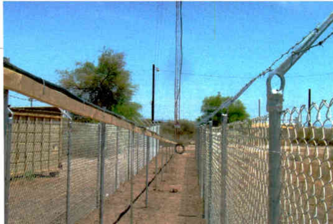
Fig. 5: Here's a means of protecting cable against vandalism when it can't be buried.
