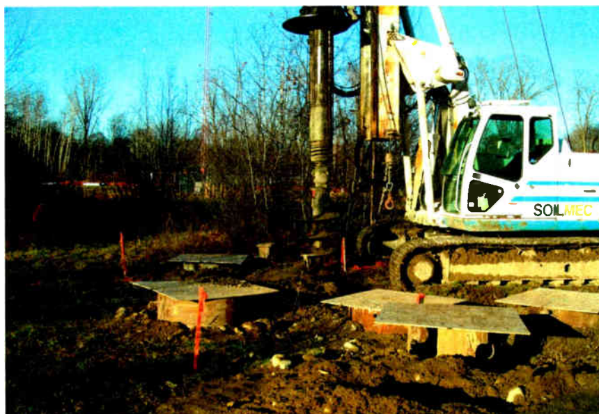
Site work at Clear Channel's AM triplex in Boston. Opponents of the ratchet clause say its effect is to discourage AMs from making antenna system improvements.
