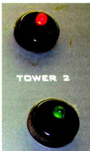
Fig. 3: Broken filaments are eliminated by converting to LEDs for phasor indicators.
