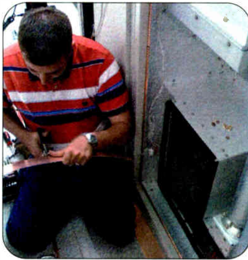
Chief Engineer Chris Dusterhoff installs ground strap on a new Harris transmitter.
