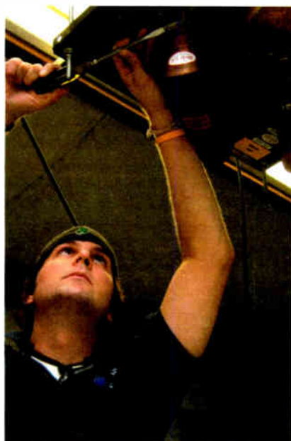
Jasen Bragg, DOE and IT director for Cumulus Media of Shreveport, works on a switch at a Gap facility.
