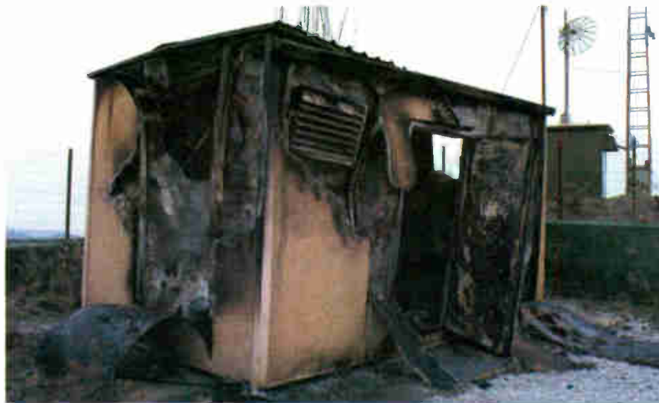
Fig. 3: The building in Fig. 1 after Mother Nature got done with it.
