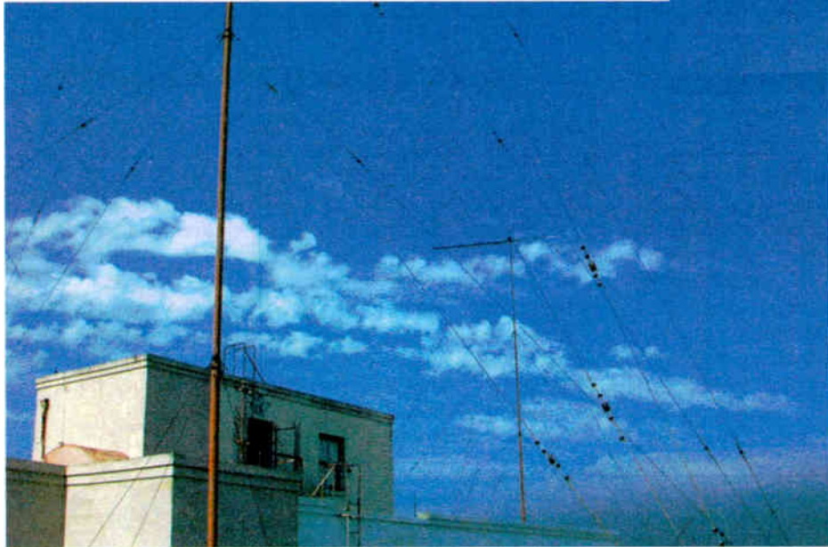
A close-up view of the former KGFJ/KYPA inverted L flat-top antenna. The north end of the antenna is close to the center of the picture.
