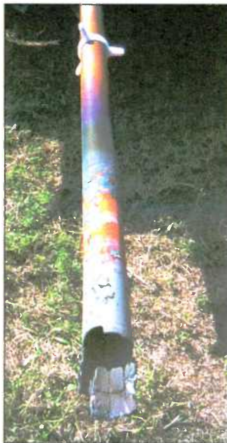
Fig. 2: The real damage occurred some 70 feet below the top bay. This inter-bay line was melted by the sustained RF arc.
