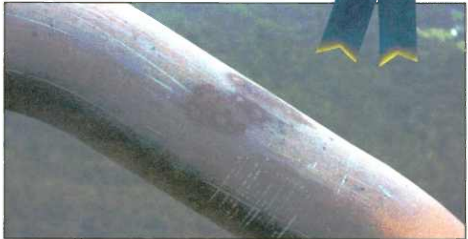
Fig. 1: Lightning hit this top FM bay, pitting the surface and causing an arc within — note the discoloration due to heat.
