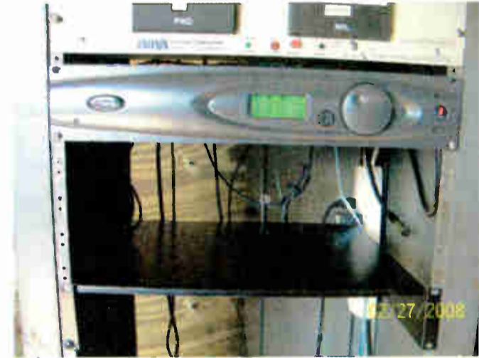
Fig. 3: Rack shelf in place after the exciter is removed.
