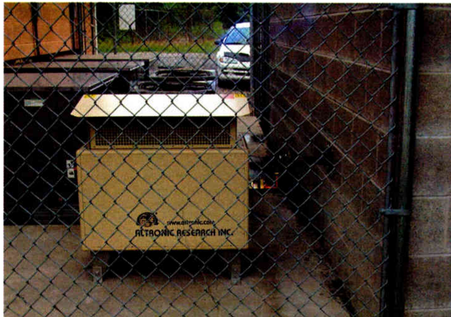
A reject load is required for high-level combined FM systems. Outdoor loads like this help with costs by keeping the heat outside.
