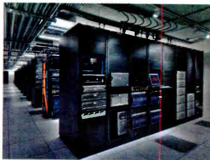
Rack Room/Tech Core
