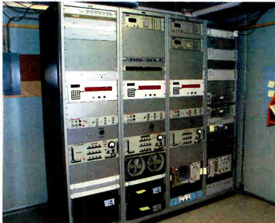
The time code generation room at WWV. This is a shielded room that holds the three — primary, secondary and tertiary — time code generators and digital announcers used for the WWV stations.
