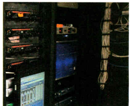
Pictured is our installation in the New York studios of Univision, integrated by CBC Broadcasting, Inc. Photos by George Snure, CBC.
