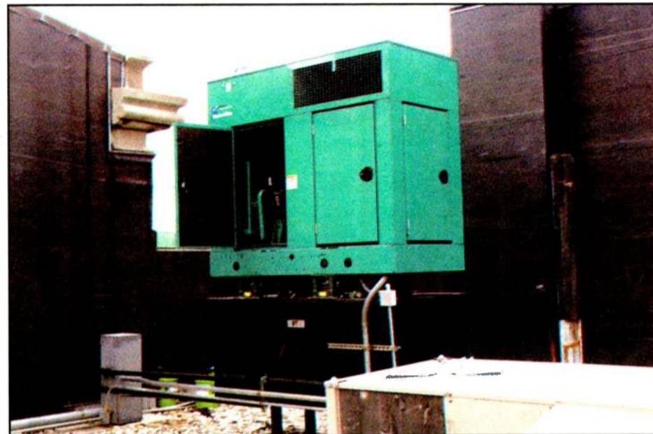
Fig. 9: The generator sits in the southwest corner of the roof, hidden by the façade.
