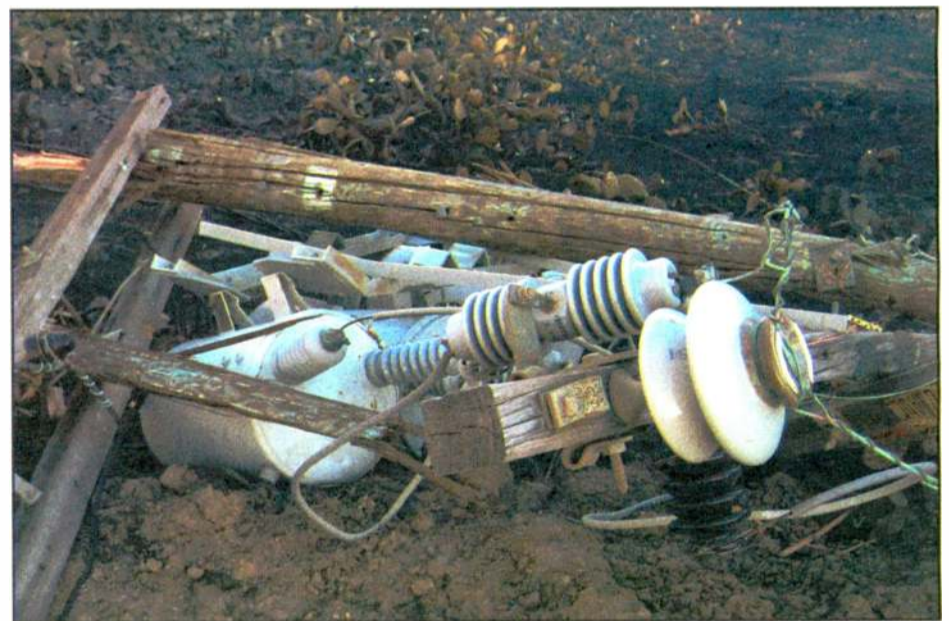
Fig. 2: KBRT's Edison transformers are in the dirt following the supporting pole's collapse in the fire.
