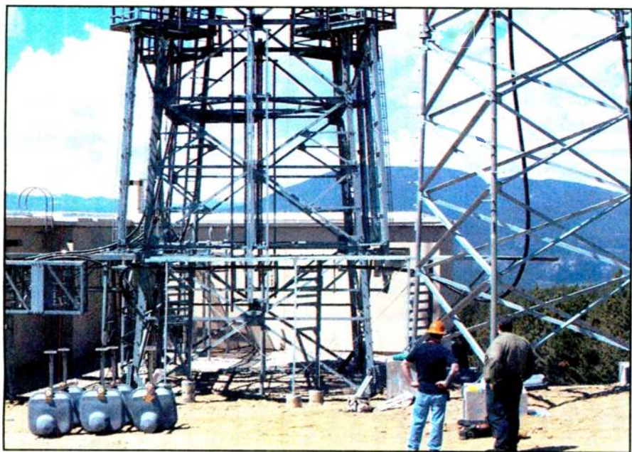
A view of the antenna bays (lower left) waiting to go up the tower.
