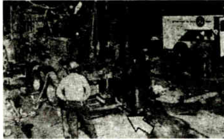
Grainy photo shows drilling rig with VM tape recorder resting on platform above bore hole and casing.
