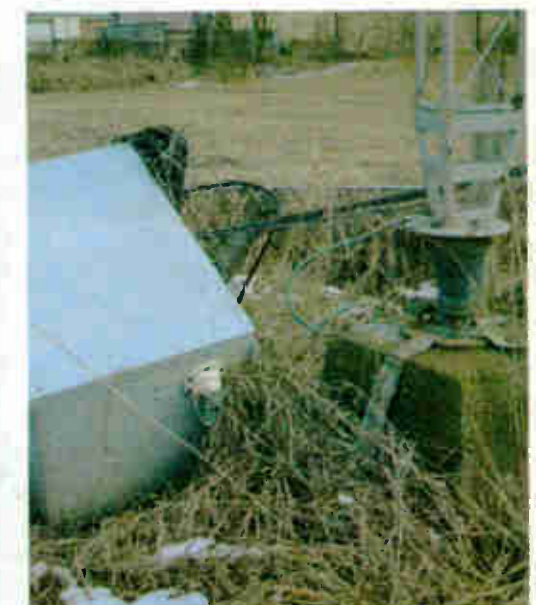
Fig. 5: Even with a toppled ATU, the antenna is still being fed!
