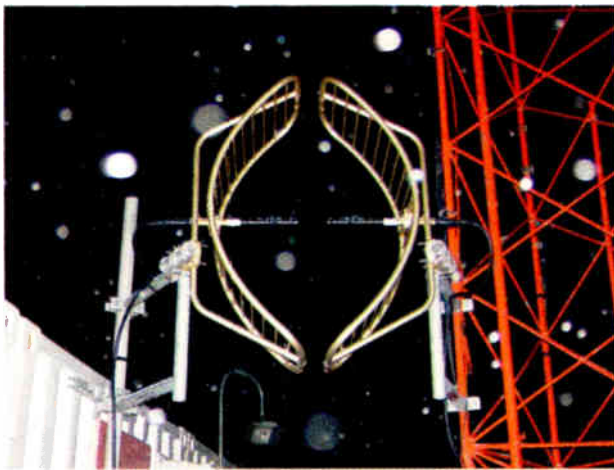
Fig. 1: Not only STL dishes but yagis can be used to couple across an AM base insulator.
