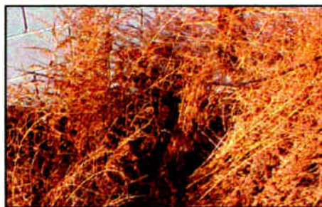
Fig. 4: Exposed cables threaten the air-worthiness of this station should fire strike.
