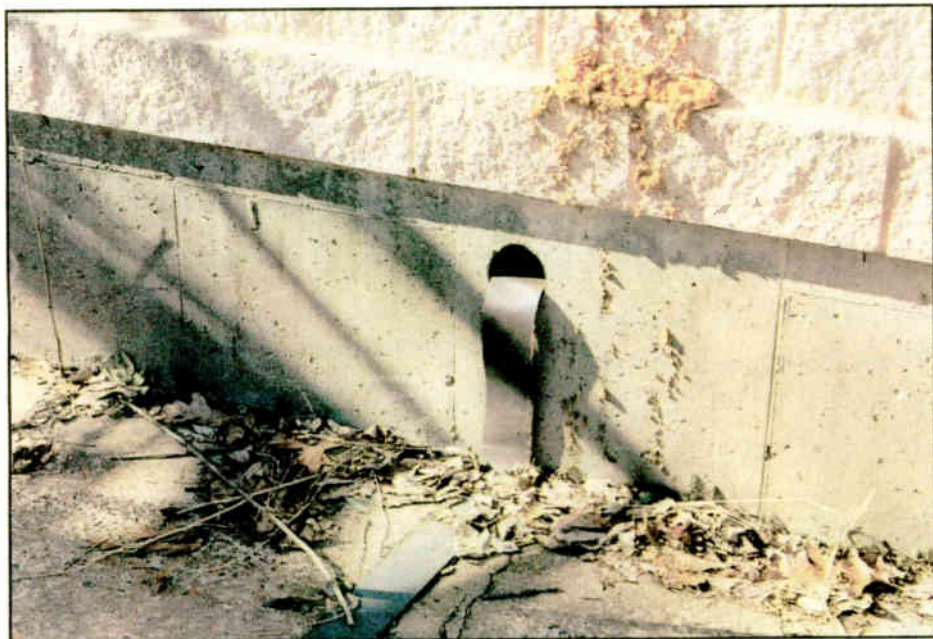
Fig. 1: This cored hole for a ground strap has been left unfilled. Hang a sign: 'Rodents Welcome.'
