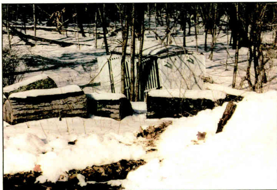
Fig. 3: A burned-out packaged high-voltage unit was abandoned so long ago that trees have grown around it. What sort of oil is left in this tub?
