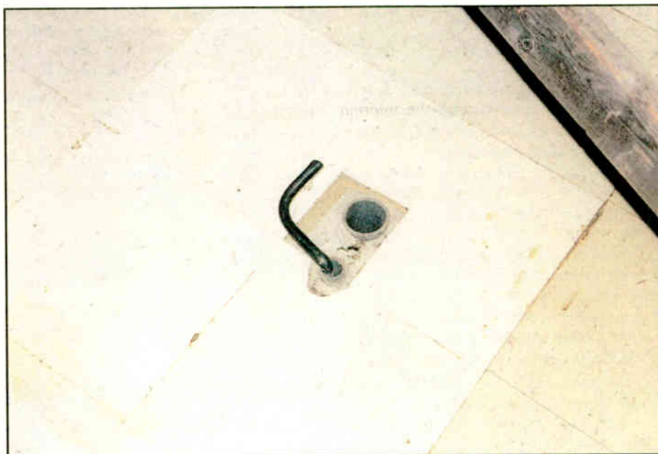
Fig. 2: This is the other end of the hole in Fig. 1. 'What goes in must come out...'
