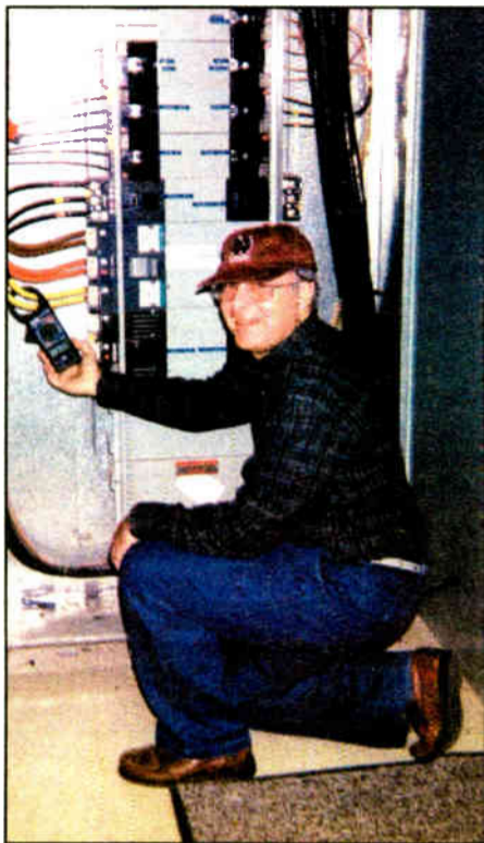
The author takes a current measurement in a 1200-amp, 480-volt distribution cabinet.
