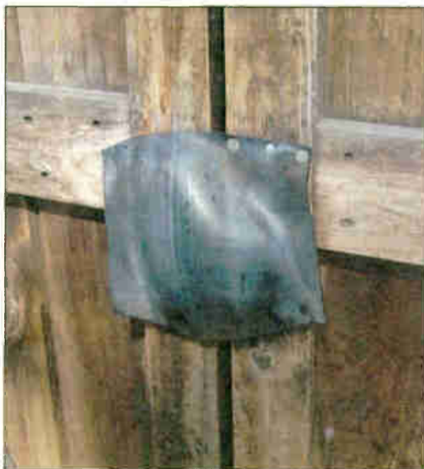
Fig. 1: Flaps cover and protect locks ... but provide a haven for stinging insects
