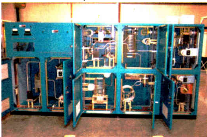
THREE TOWER AM 50kW NDA-D / DA-N DIRECTIONAL ANTENNA SYSTEM ST PAUL, MN.
