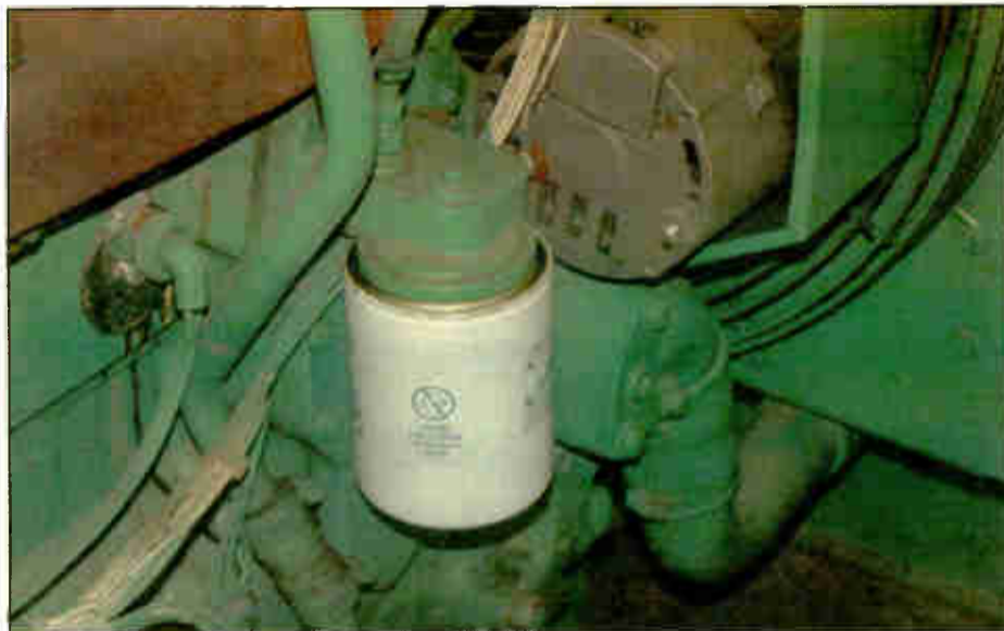
Fig. 4: As you inspect the generator body, search for leaks, especially around filters and engine seals.
