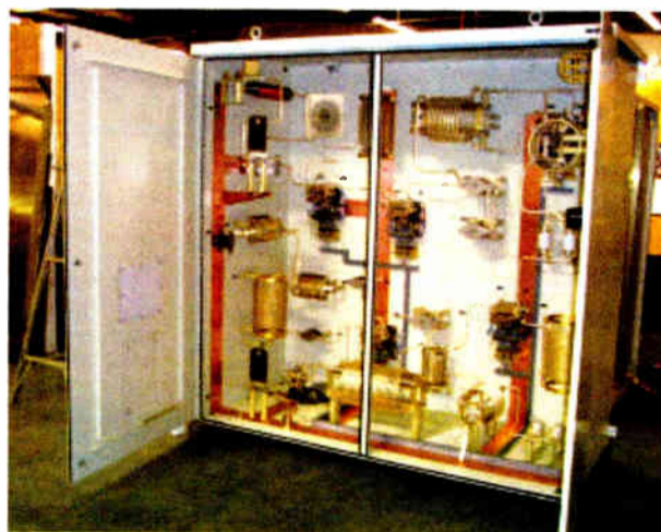
DIRECTIONAL ARRAY ANTENNA TUNING UNIT GAITHERSBURG, MD
