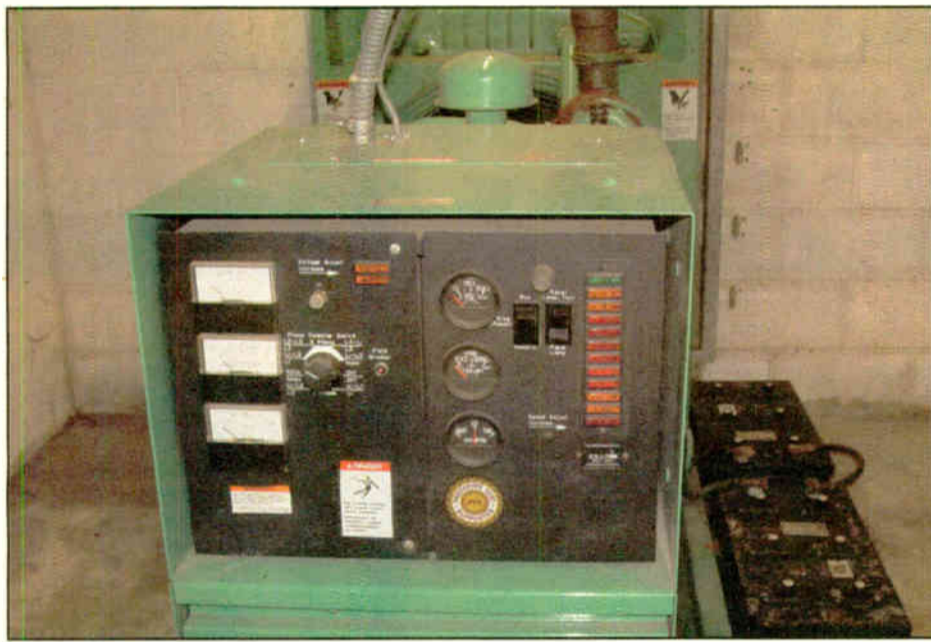
Fig. 1: Keep a log of the meters on your generator.
