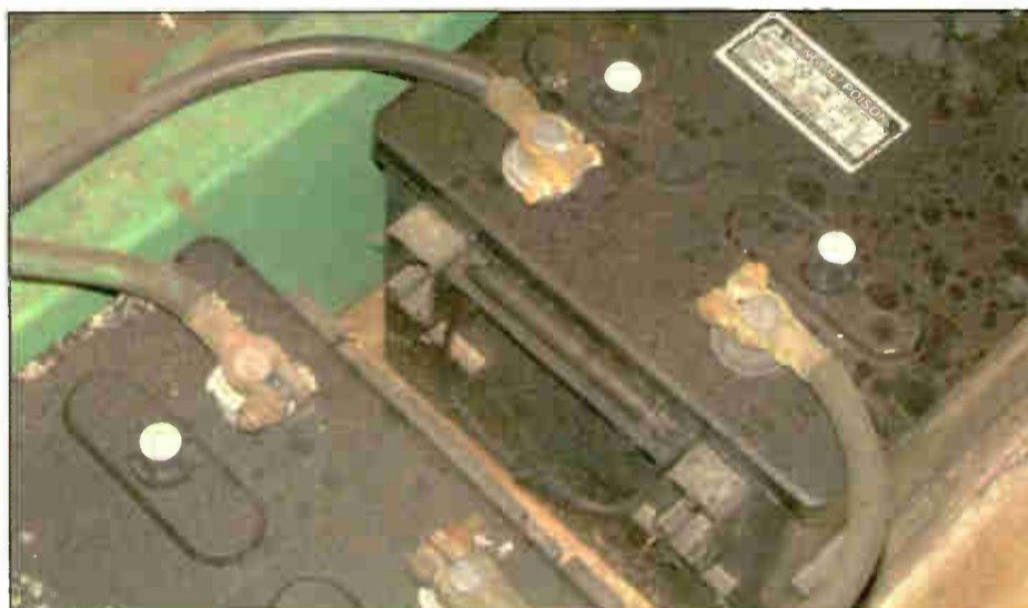
Fig. 5: Pretend it's a car: inspect battery cables, remove corrosion from the terminals, tighten connections.
