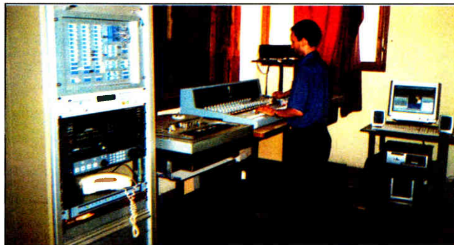
Hamza Bachiri, technical director of RTM's regional station in Oudja, tests the AEO Mixing and Automation System.
