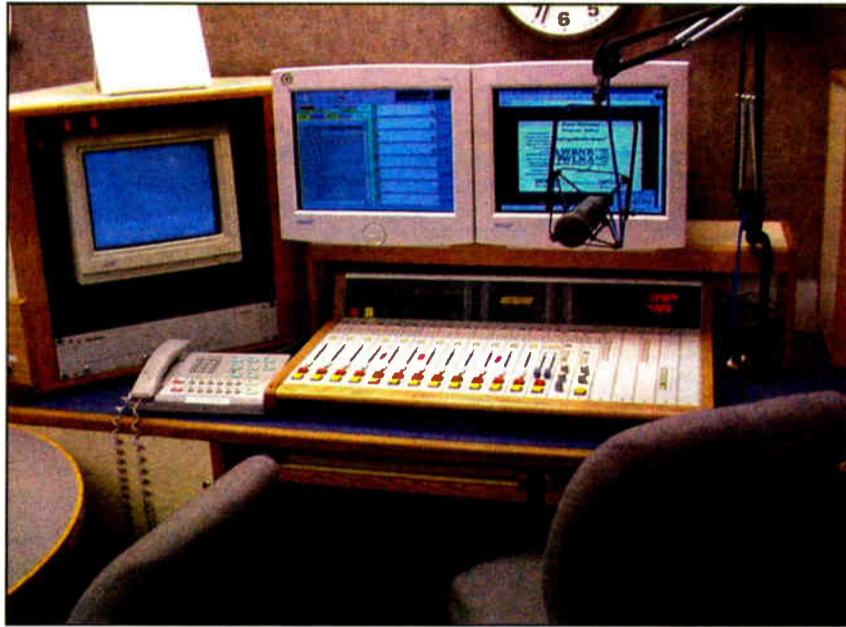
The BE Vault 2 efficiently networks clusters of stations.
