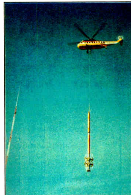
Mark Humphrey of Radio One took this photo of WPSG(TV)'s antenna being airlifted to the Gross Tower. The FM antenna for WMGK/WMWX is attached to the base. Another tower is at left.
