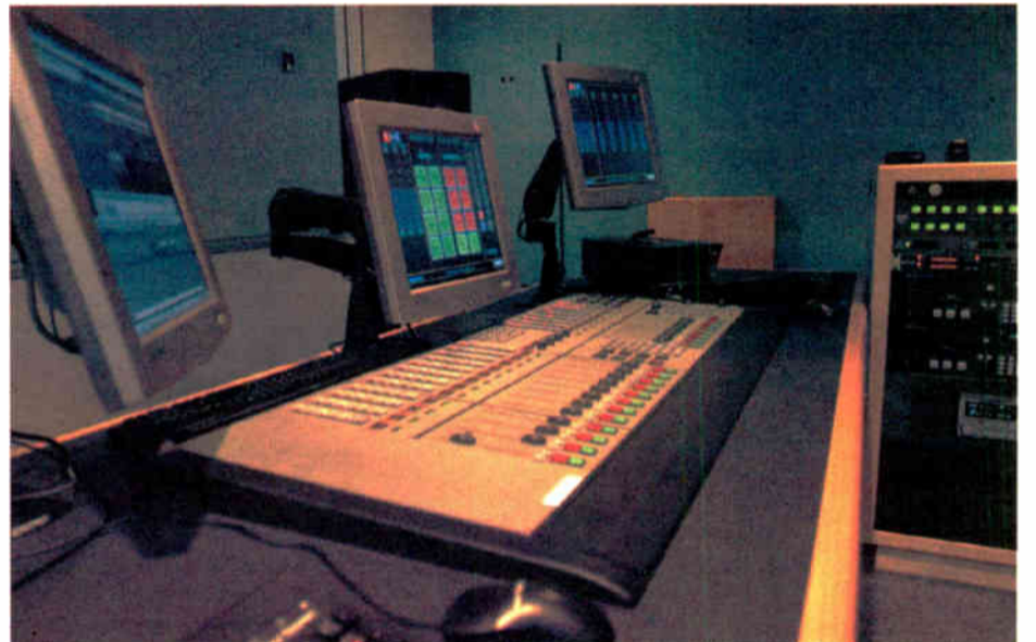
A Klotz Vadis DC II digital board interfaces with a digital network at NPR West.
