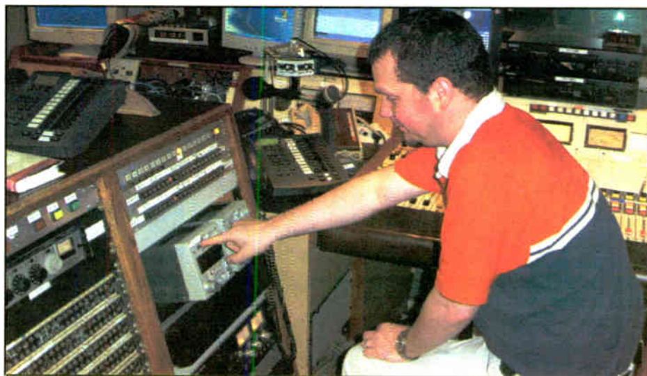
WOR operators easily switch tracks with the rotary track selector.
