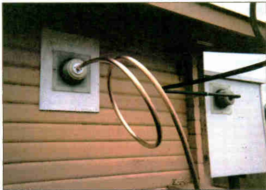
Fig 2: The external feed line is shown.
