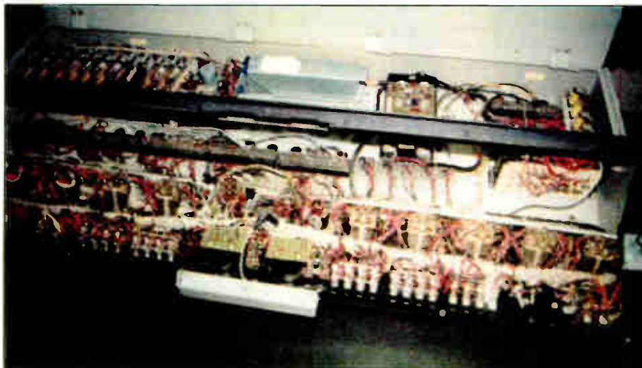
Too many previous repairs, too confusing, no reliable source for parts. The interior of the console.
