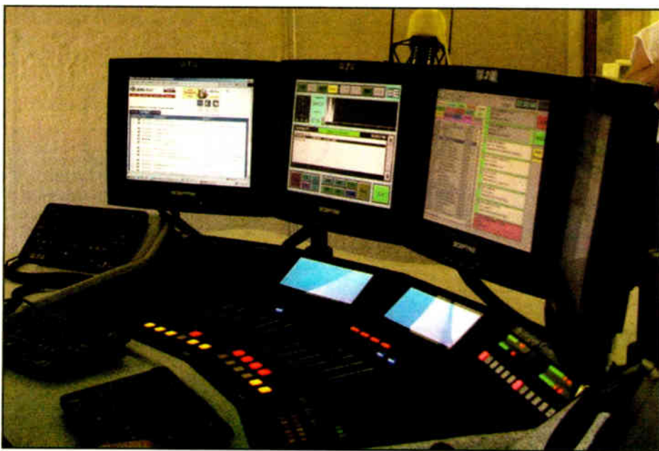
Shown is the installation at Citadel Communications in Nashville, Tenn., with the Logitek Audio Engine and Numix console controller.
