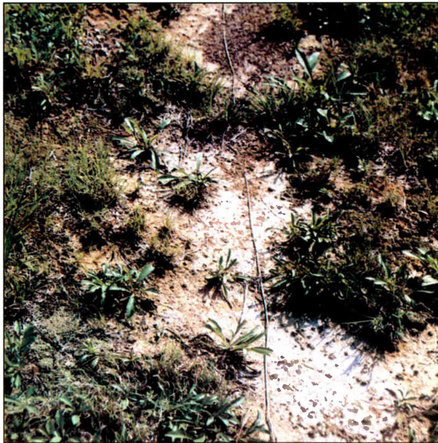
Fig. 3: Be on the lookout for exposed radials.
