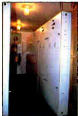
Wideband AM Diplexer Installed In Prefab Building 660KHz/880KHz 2 x 30kW
