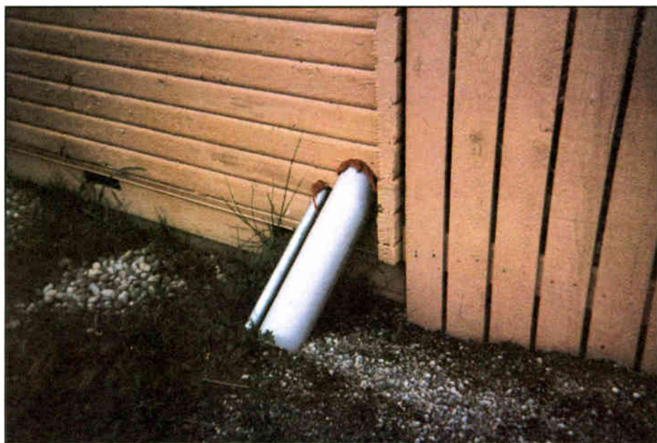
Fig. 1: Expanding foam can be used to seal coax and control pipes at tower buildings.
