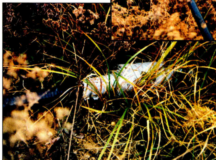
Figs. 3 & 4: The engineer tried to keep this transmission line off the ground, top, and secured the splice kit with duct tape, above. Unfortunately these temporary fixes were made 10 years ago.
