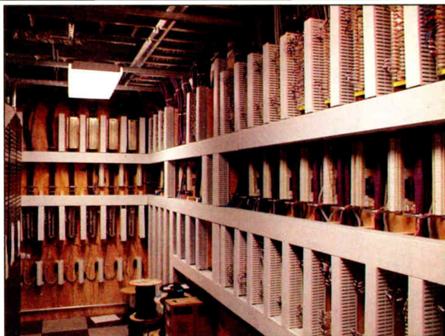
Entercom Engineering Room With Molex Wiring
