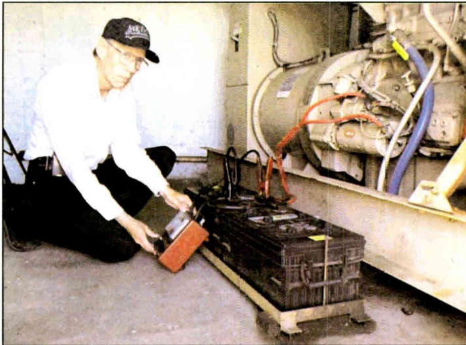
Art Lebermann runs a load test on the batteries for the 275-kW diesel generator at KGO(AM), San Francisco.
