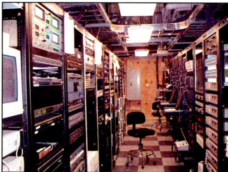
Entercom Engineering Room Rack Layout
