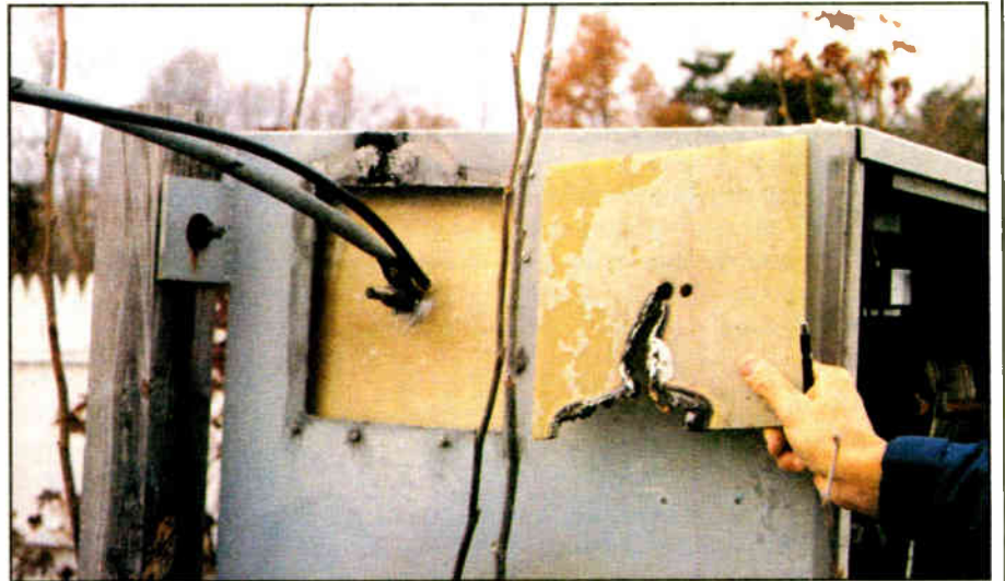
Fig. 2: The output insulator on this coupling network burned to the case, and eventually self-extinguished.
