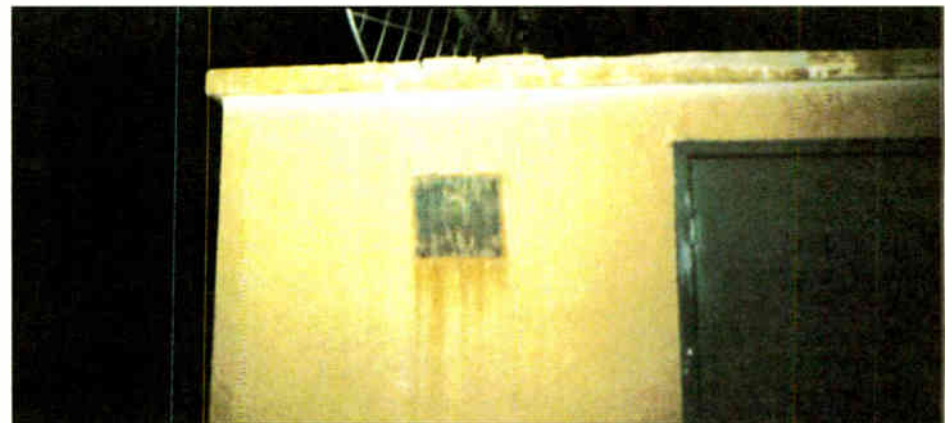
Fig. 3: The roof is sealed but the unused vent lets water through.
