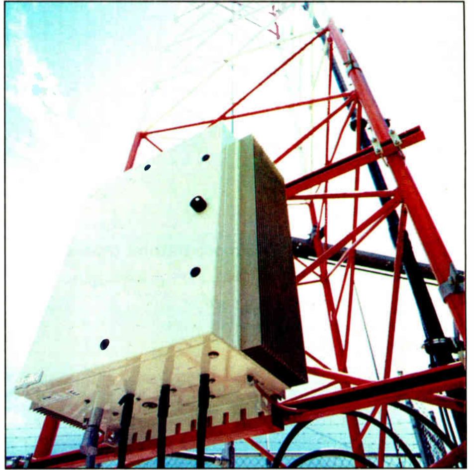
AirSite Base Station on an antenna tower
