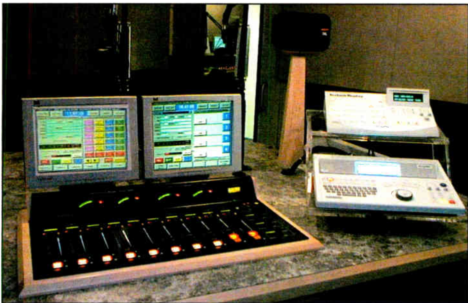
Radio Super Estrella on-air studio with Logitek's console control surface
