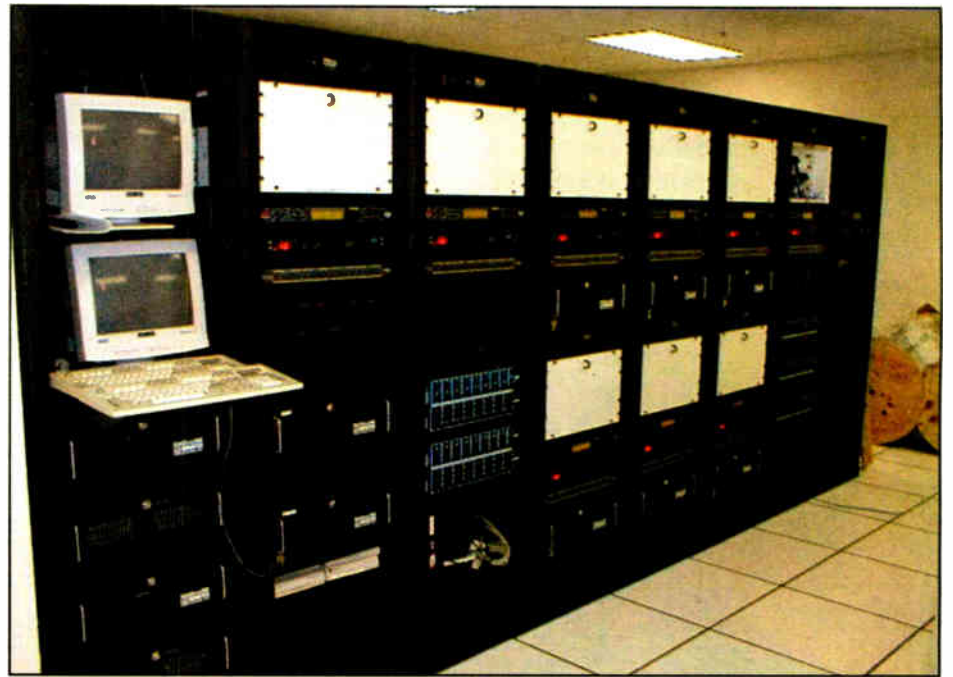
EXCL's master control/uplink rack room with 10 Audio Engines
