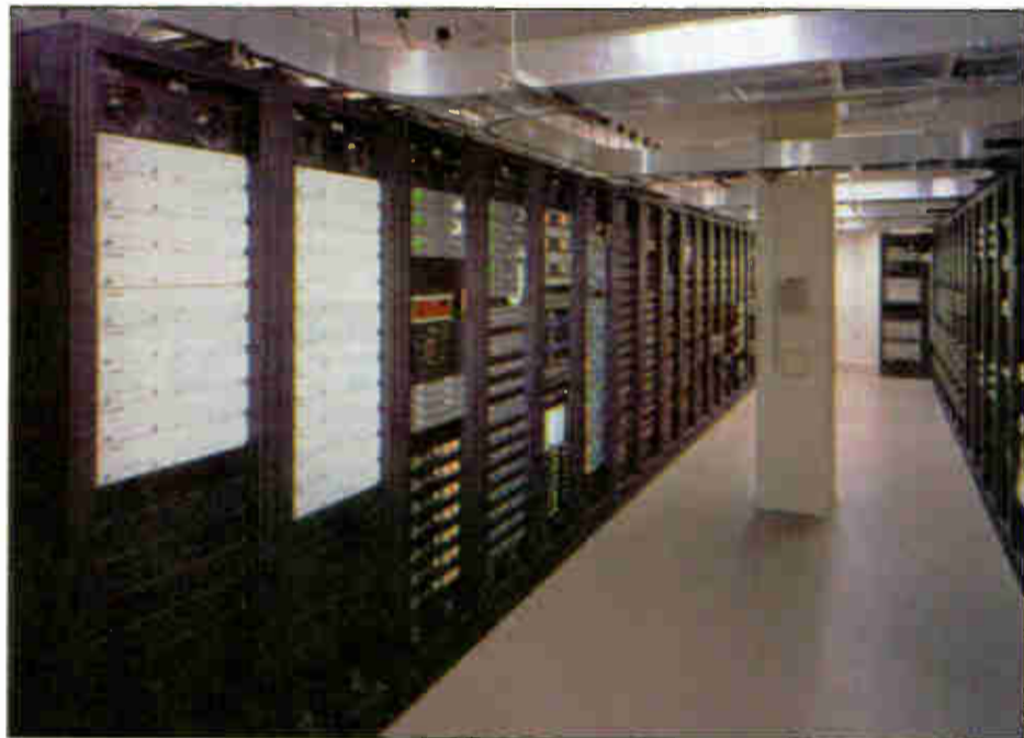
The Main Rack Room
