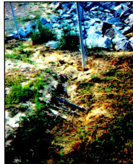
Figure 3: Exposed transmission lines are accidents waiting to happen.
