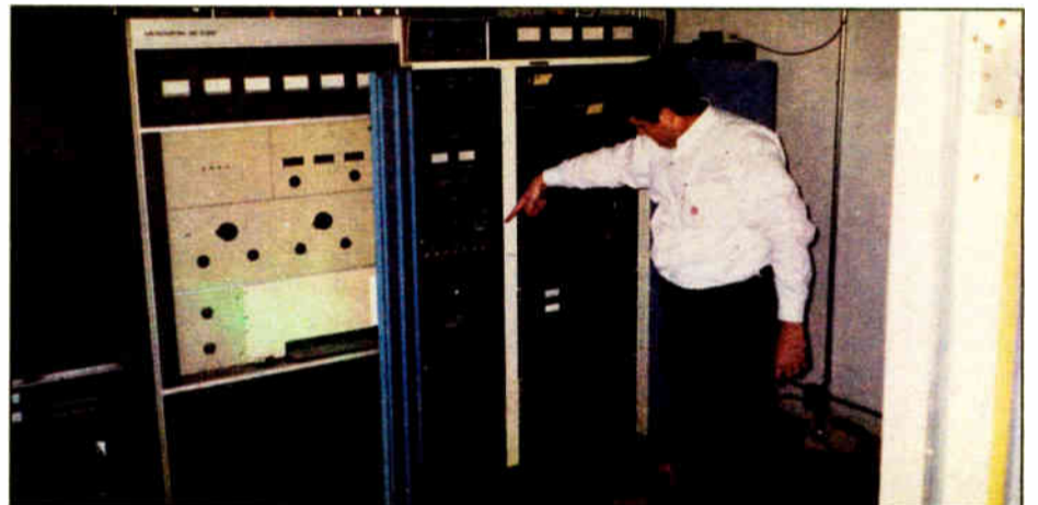
Paul Matthews points to the water line on the Harris FM 20K transmitter. The exciter is visible 12 inches below the water line.
