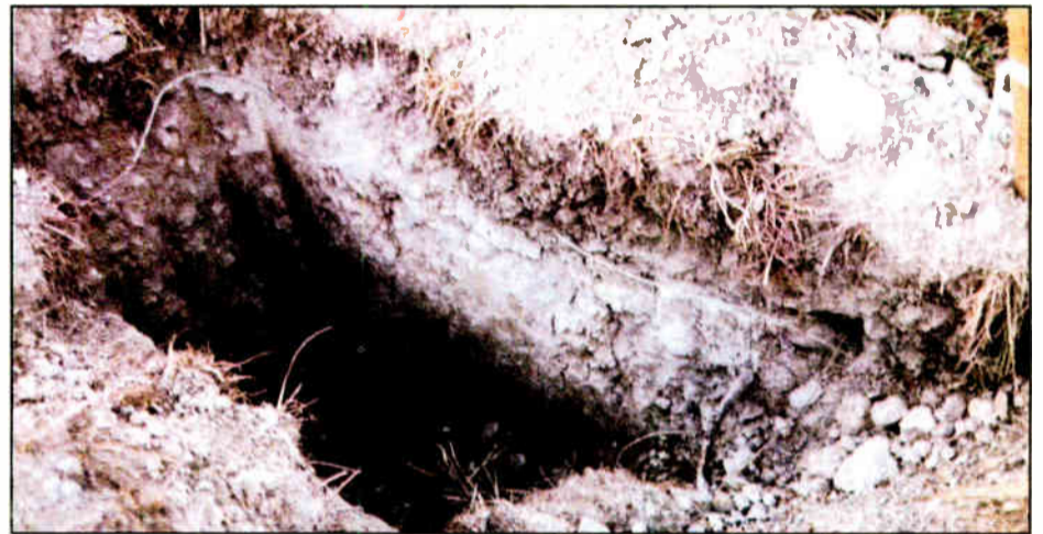
Figure 1: Don't let a backhoe ruin your day by ripping up your ground system — personally supervise any construction at your transmitter site.
