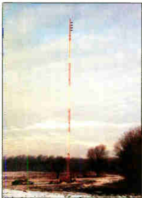
The new tower is three times as tall as the old one.
