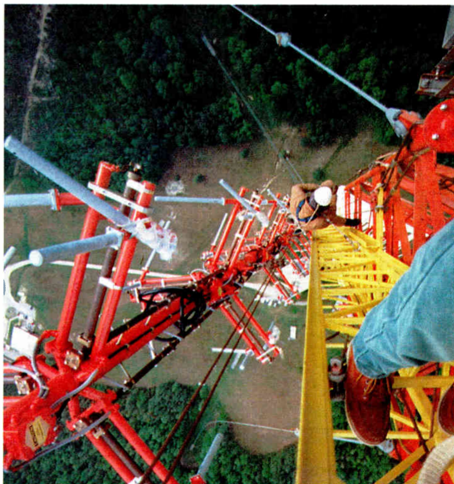
Figure 2: It's 'element-ary.' Installation of some antenna elements must wait until after the antenna is safely rotated around the yellow gin pole.
