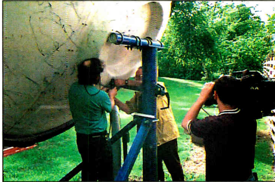
Vermont Public Radio CE Rich Parker, left, and Contract Engineer Ira Wilner prepare to move the dish.
