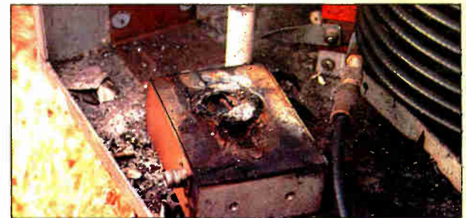
Figure 2. Loose connections can have catastrophic results.
