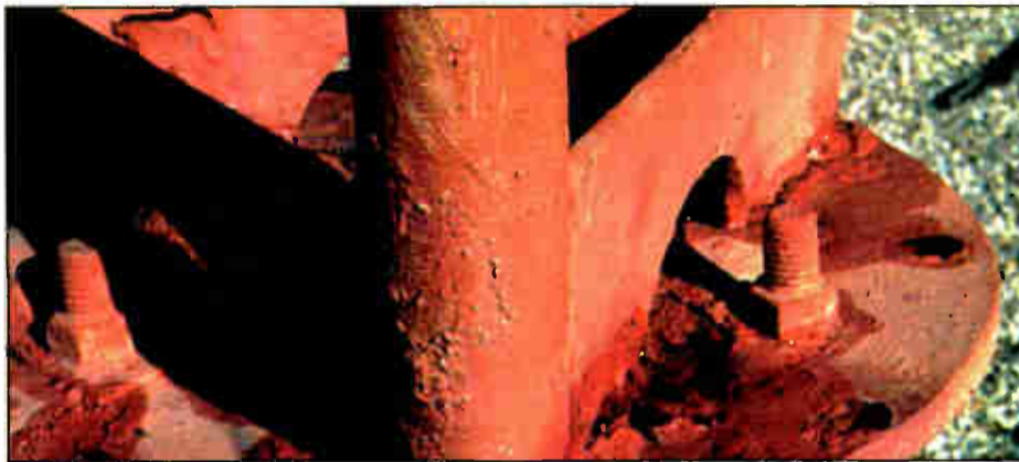
Figure 1. Water does its damage to a tower base.
