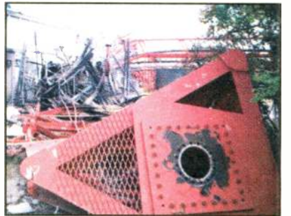
Part of the Top of the Toppled Tower
