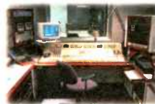
Integrated Systems Our turnkey solutions cover your entire project—from design through installation.
