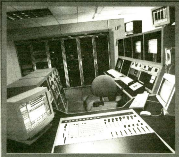
The Master Control Studio, shown right, is one of seven Arrakis studios in Sony's Manhattan network origination center for SW Networks.
