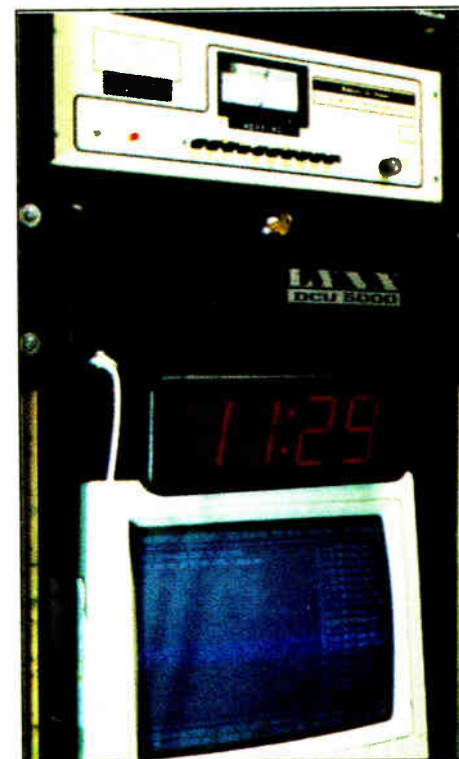
The LYNX installed as part of an FM translator
