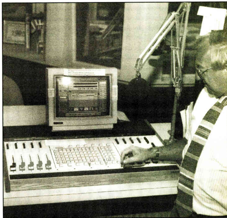
Larry Wilkins with the Gemini panel, installed in a Gem6 console.
