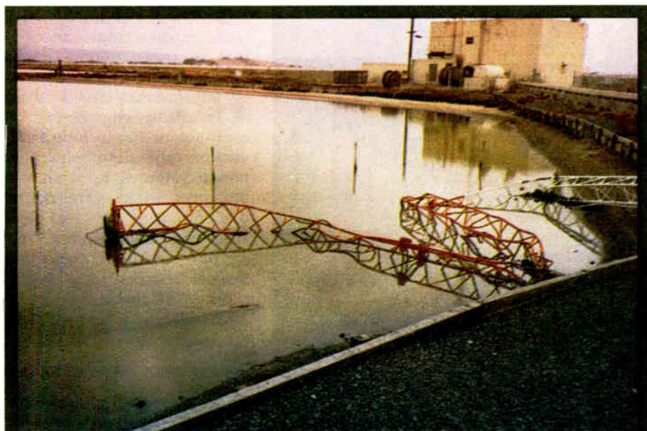
KGO's crumpled tower showed that it fared worse than KABL.
