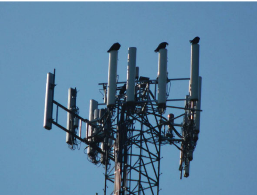
This lightweight t-frame mount is loaded with LTE equipment. It failed at >200 percent when analyzed for the existing loading. A full mount replacement was recommended.
