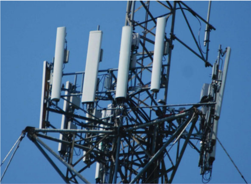
With this lightweight t-frame mount, the proposed loading consisted of only remote radio units. The mount failed at >200 percent when analyzed. A bolt-on prefabricated modification was proposed to reduce mount stress rating to <100 percent.
