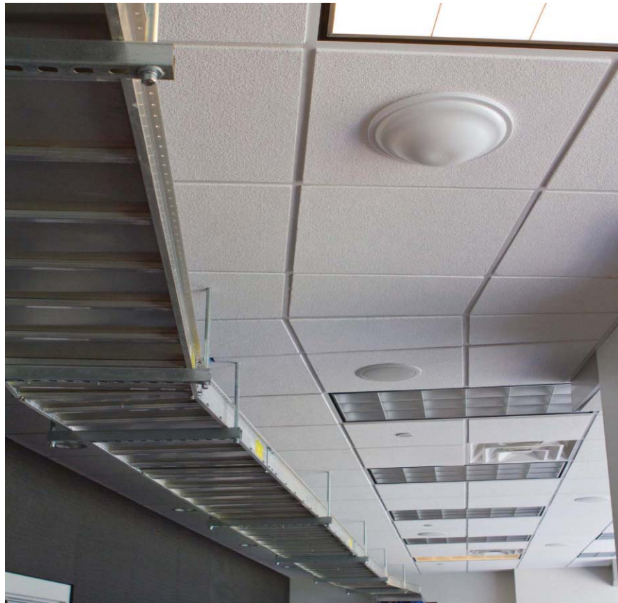
Figure 2: Ceiling-mounted DAS antennas require little maintenance, but they may be inadvertently unplugged during other work in the area.
