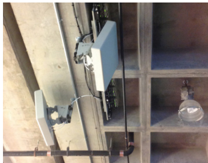
Indoor antennas for cellular service.
