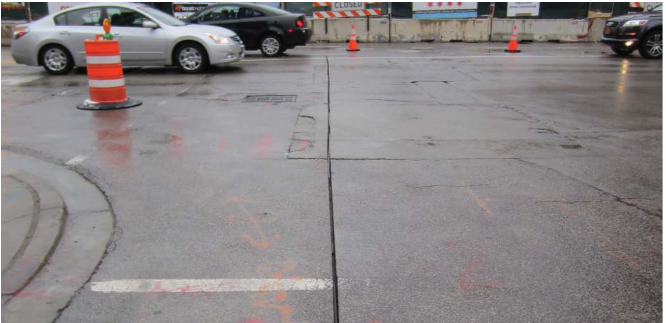
A lengthy saw-cut microtrench only needs traffic barriers during the saw cut and final microduct placement, whereas traditional inner duct installation requires a wider trench and traffic control barriers or both for the duration of the installation.
