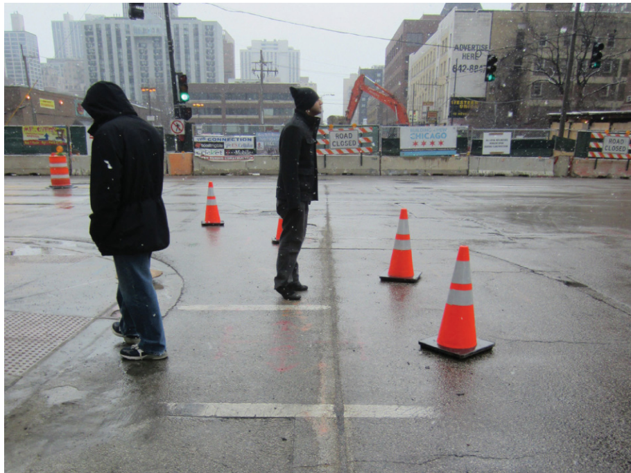
Restoring the trench after placing the microduct often can be done in a single pass that includes placing restoral material and a topcoat of concrete or asphalt.
