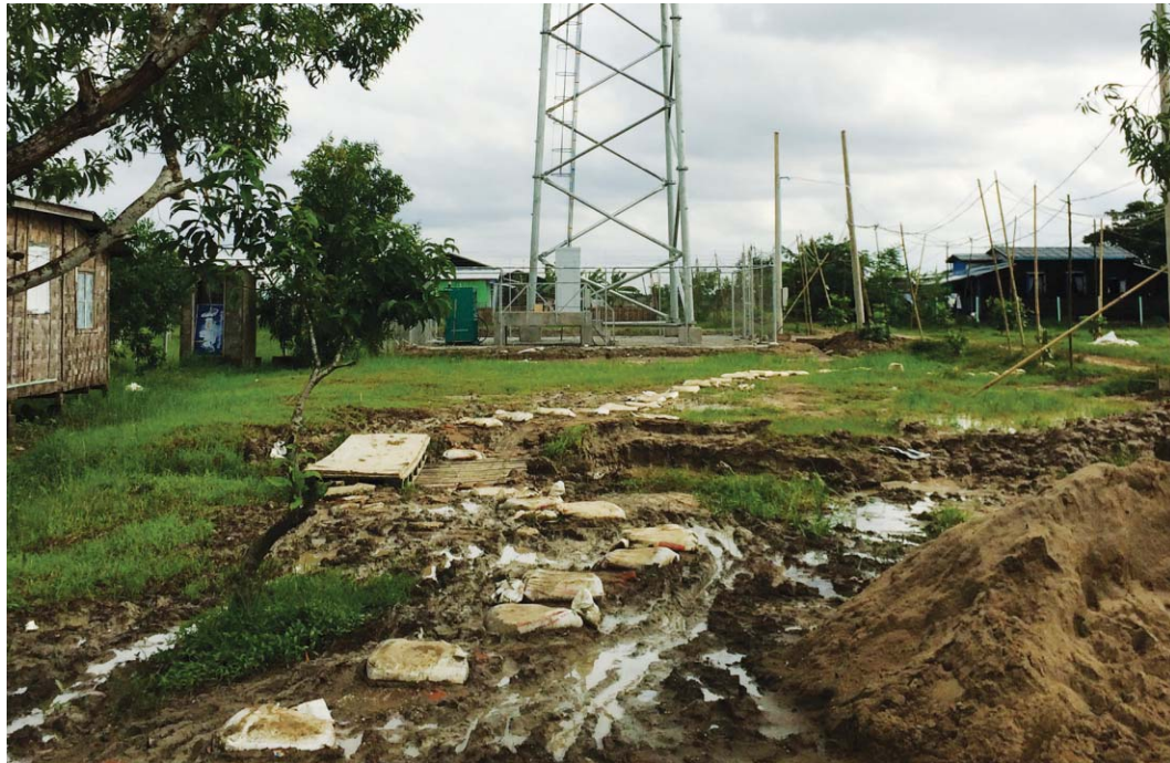
Mobile networks powered by Cummins have been installed in parts of Myanmar where even roads have not reached yet.
