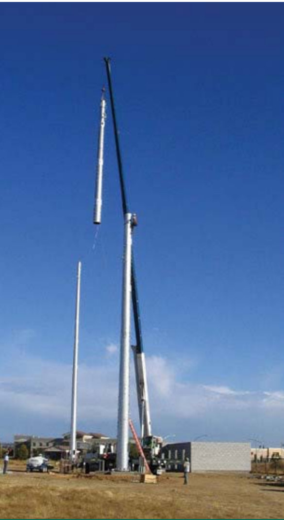
A crane lifts the west tower's third and final tower section into position.
