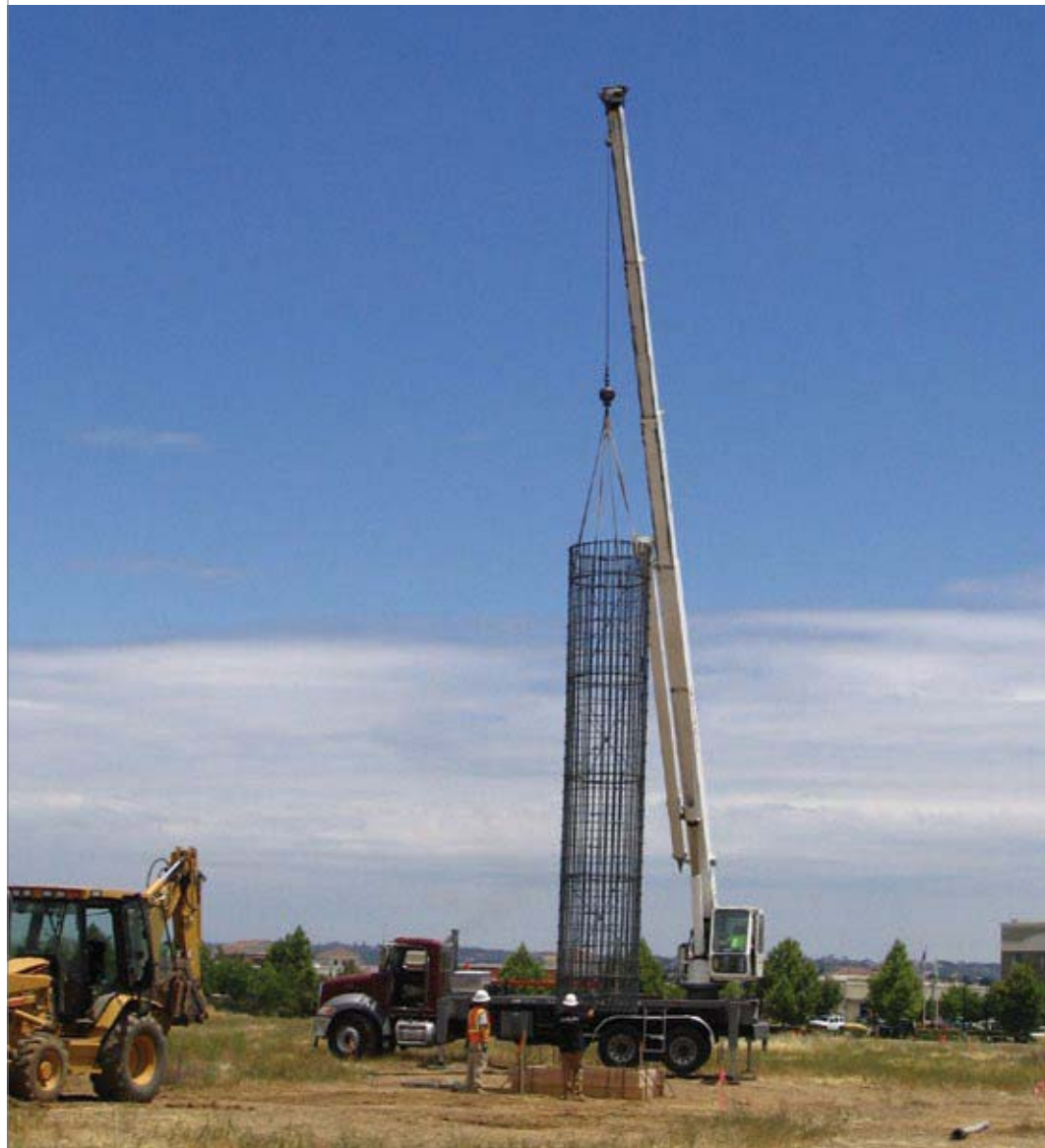
Just prior to concrete being poured, a crane lowers a reinforcing rebar cage into the east tower's foundation bore.
