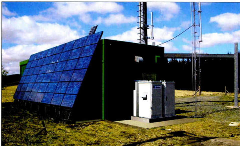
At this telecommunications site, an integrated fuel cell system works together with a solar panel array to provide extended-run backup power.
