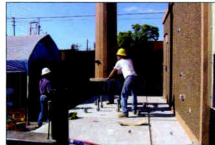
Prior to the end of the day, the monopole is stacked, and the installation of equipment begins.
