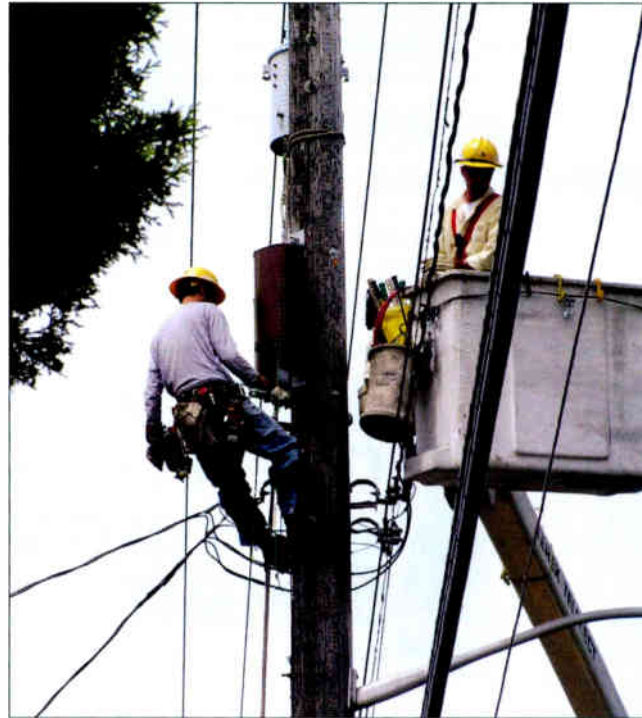
Workers install part of a distributed antenna system on a utility pole in Seattle. Crown Castle used both panel and omnidirectional antennas at the remote antenna nodes depending on the surrounding terrain.
