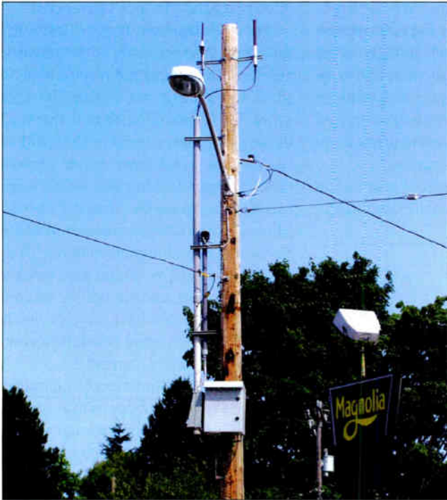
A remote access node in Seattle includes two omnidirectional antennas placed in a favorable position at the top of a light pole that has no medium-voltage distribution lines to obstruct antenna placement.
