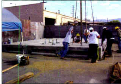
Work to place the precast foundation began at 8 a.m., and at 9 a.m., the last block of the foundation is being set.
