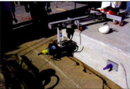
By 10:30 a.m., the post tensioning has reached 100 percent, and the foundation is complete.
