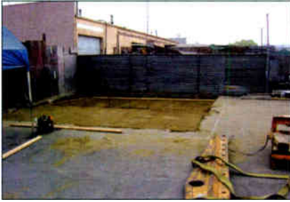
A view of a prepared site shows conditions just before the precast foundation is placed.
