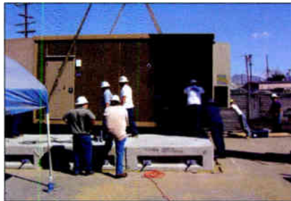
By afternoon, workers set, anchor and ground the shelter and the monopole.
