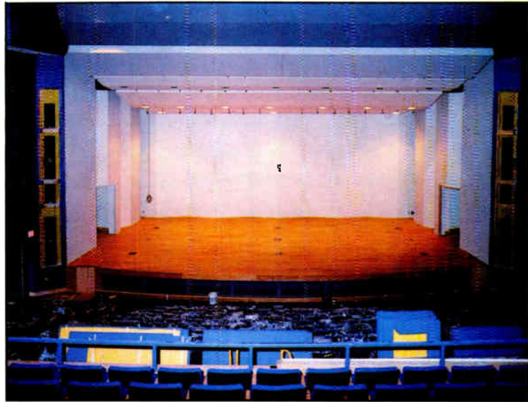
Example of an American Sound install in progress. The central cluster is hidden behind a grille centered over the stage. At the rail are acoustical panels to be hung. The walls are fabric covered fiberglass panels. This is a Jaffee Acoustics design.
