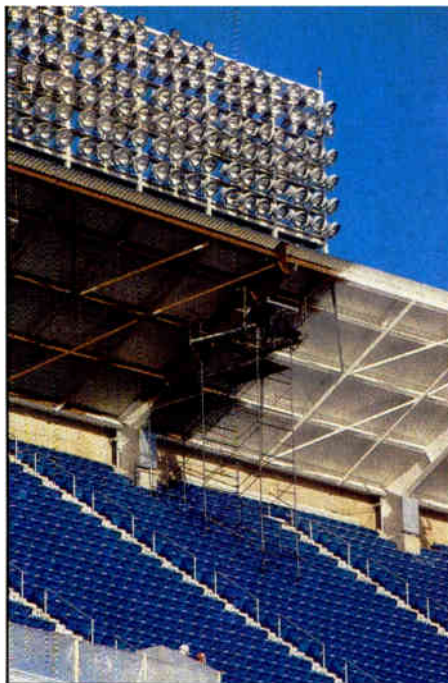
The hanging of the Upper Deck clusters is not a job for the faint of heart.
