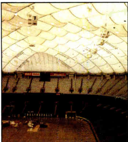
High-Directivity loudspeaker arrays were used to improve speech intelligibility and fidelity at the Hoosier Dome in Indianapolis.
