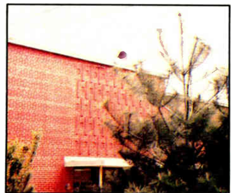
Training building speaker. Some of the cables shown are for the PA system.
