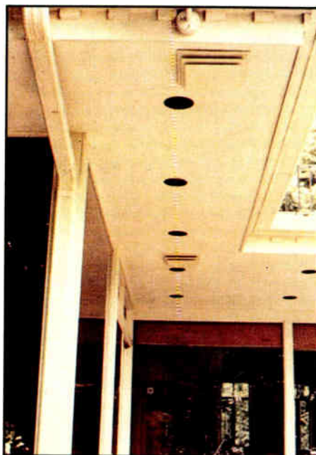
An example of Rosen's speaker used in the ceiling of a residential installation.
