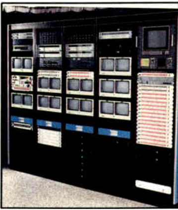
Installation at off-track betting parlor in Lancaster, Pennsylvania includes QSC equipment.
