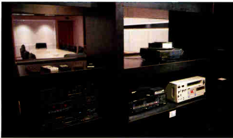
The integrated Audio/Video equipment room for Stone, August, Baker.
