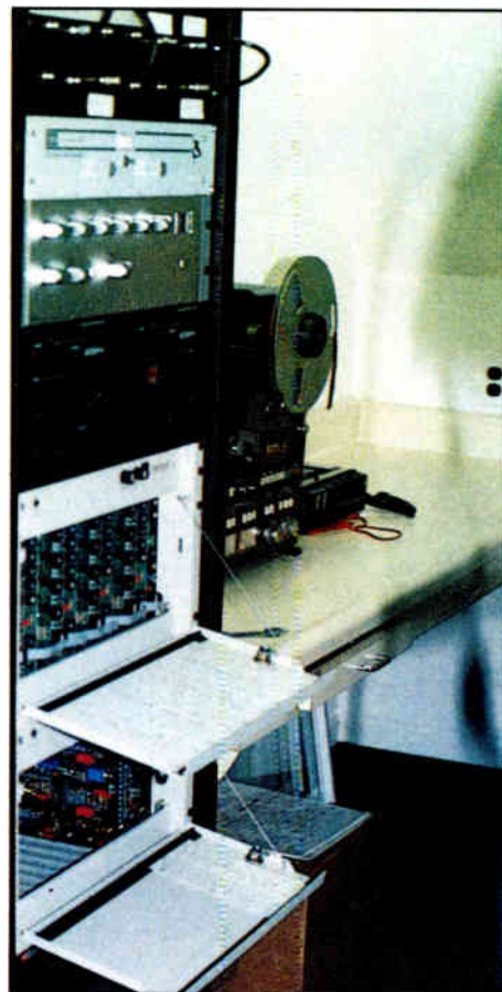
This rack features the Tandem IRP System 41, which was crucial to the Salem Baptist Church installation.
