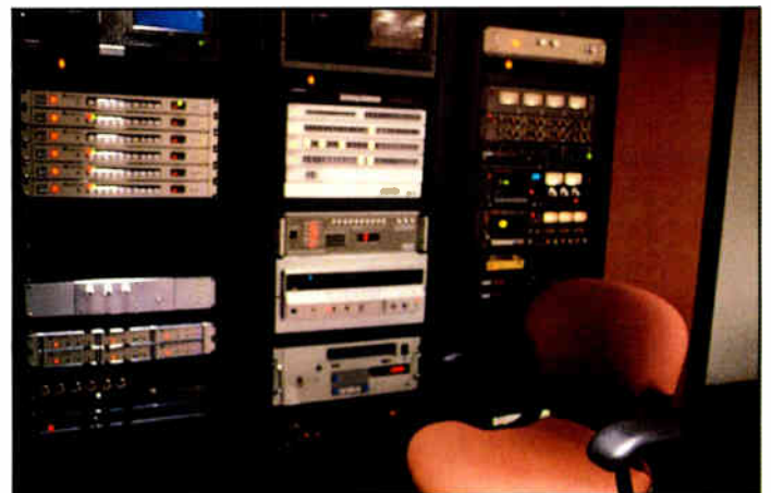
The control room for the main studio/theater.
