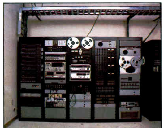
Amphitheater control room rack at Bonaventure.
