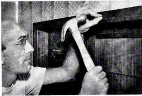
20 A final step is to frame the music wall with molding. Choose a type to blend well with other furnishings, miter the corners and nail the strips flush to the exterior plywood facing. Finish all exterior surfaces as desired.
